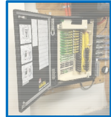
FDH Houses Splitters
