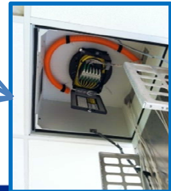
Consolidation Point Zone Cabling
