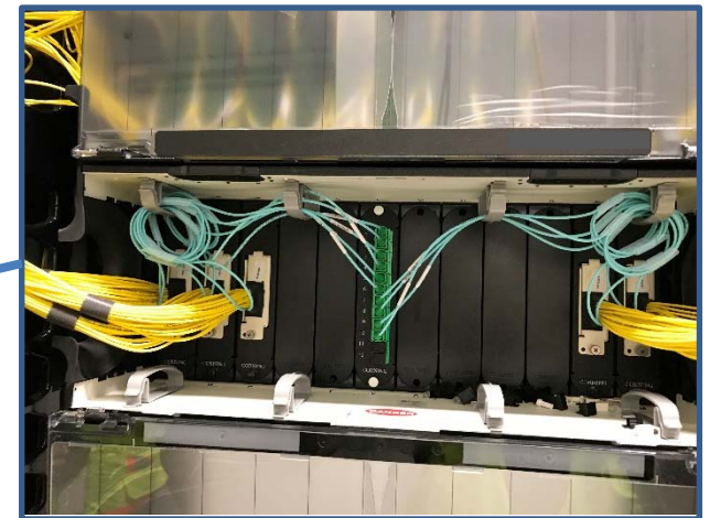
Rack-mount fiber enclosure with splitters
